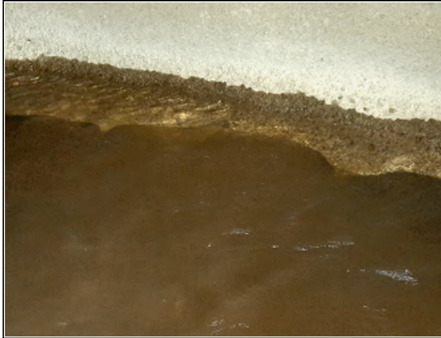
Undermining of concrete arch springline at rehab project
