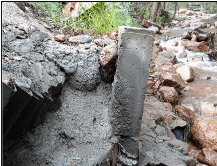
Southwest wingwall displaced, rotated
