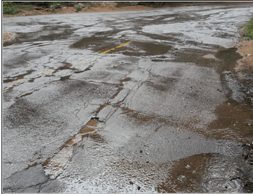
Asphalt roadway surfacing deteriorated - requires maintenance
