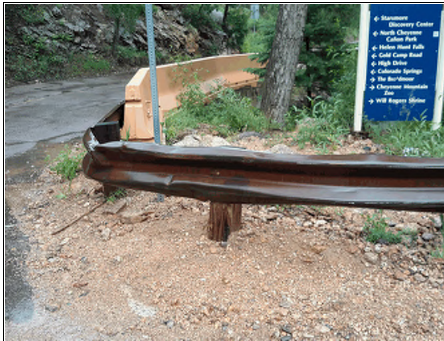
Damage at southeast guardrail
