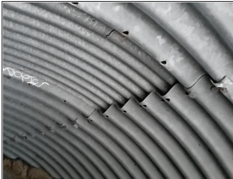
Missing bolts top of CMP plate arch. Seam separation of plates.
