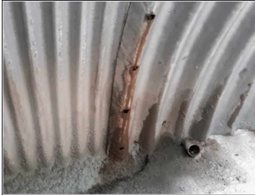
Rusting in CMP arch culvert bolt holes
