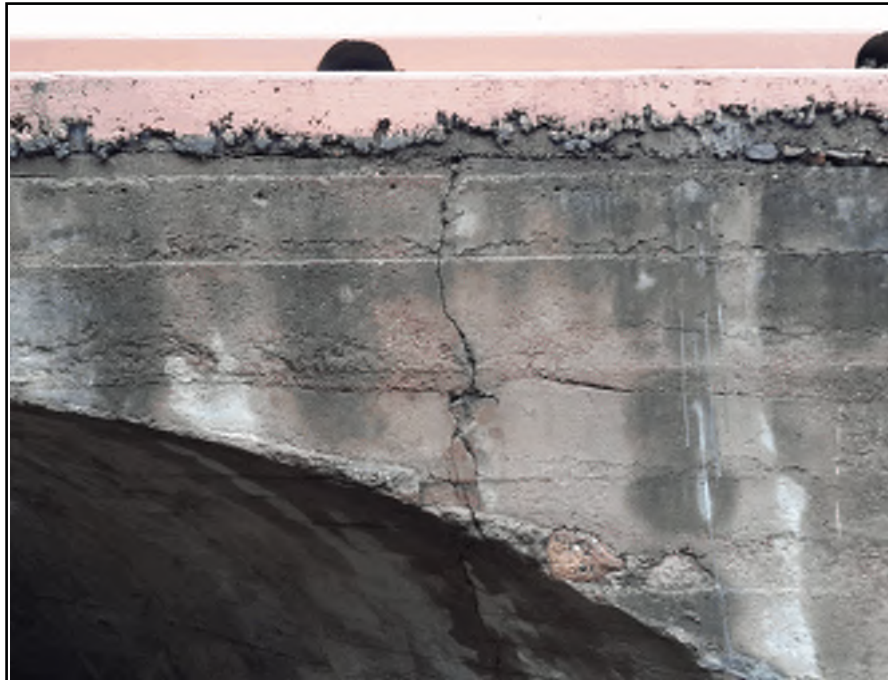
Crack in downstream headwall
