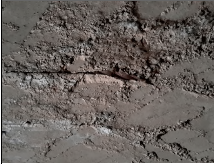
Exposed reinforcing in concrete arch
